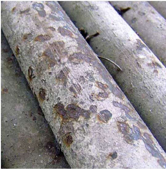
B) Scale allows corrosion to develop unnoticed on these tubes causing localised pitting but also general corrosion over the entire tube. (13)
