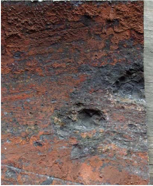
A) Localised corrosion in the form of severe pitting. This boiler barrel plate was reduced to less than \frac{1}{4} of its original thickness by corrosion.(15)
