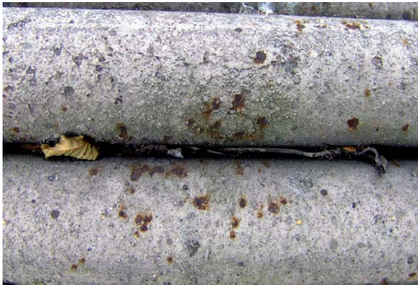
B) Less severe scaling than in 1A but none the less there is scale. These tubes had been in the locomotive in question for just 4 years and that locomotive had been on a water treatment regime, but clearly an inadequate one with scale at least a millimetre thick in places. (13)
