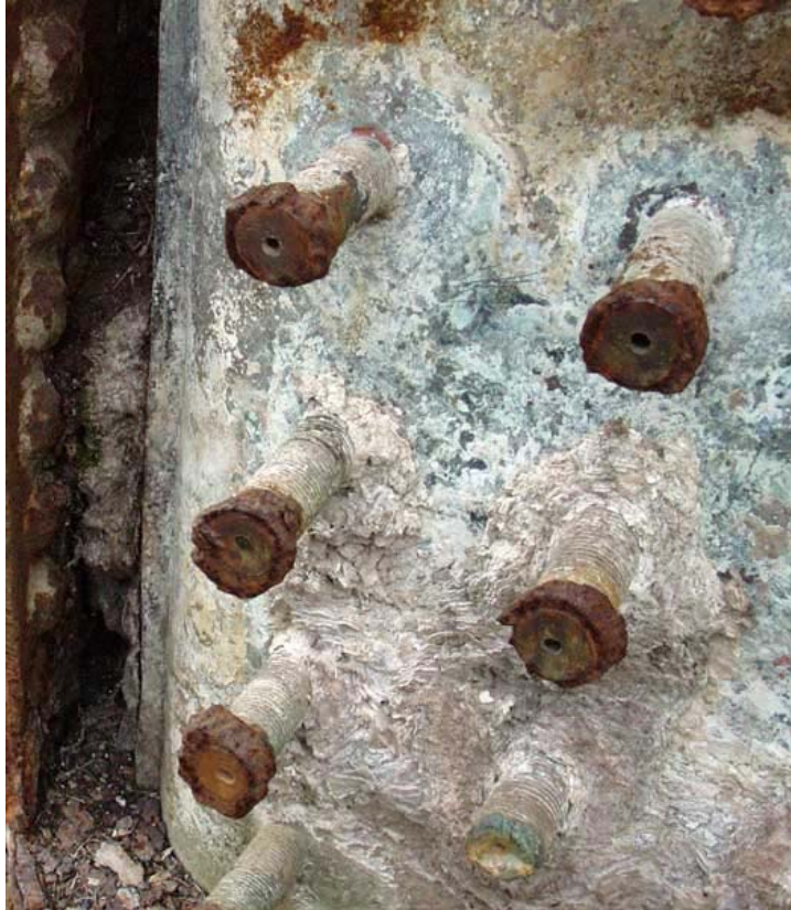
A) A boiler where scaling was so bad as to totally impede water circulation for the bottom 6" of the firebox. Not surprisingly the inner firebox was deformed.(23)
